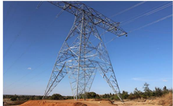
400 kV Transmission line
